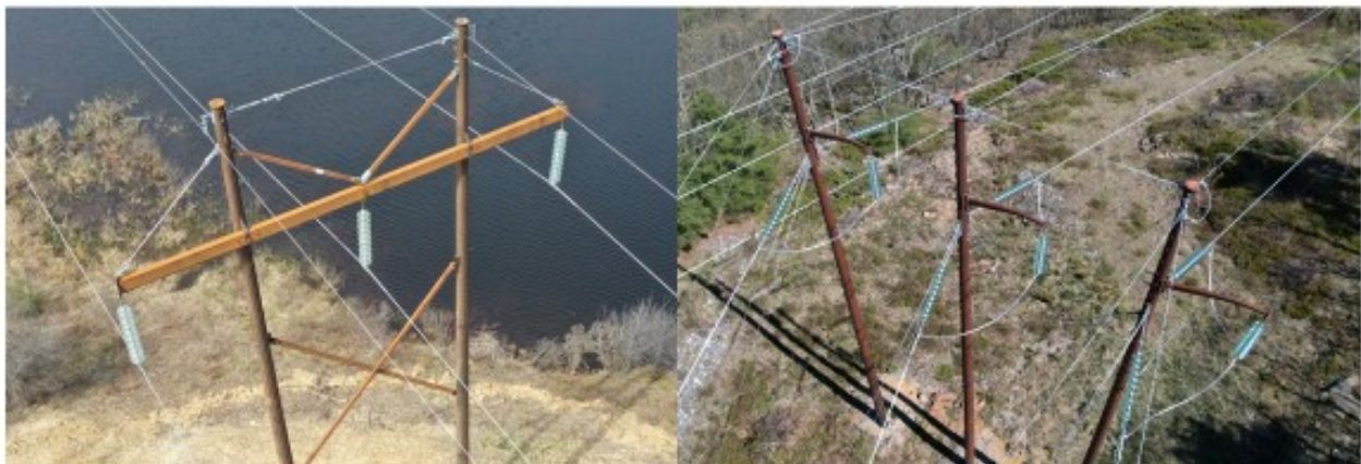
“H-Frame” structure with three insulators
