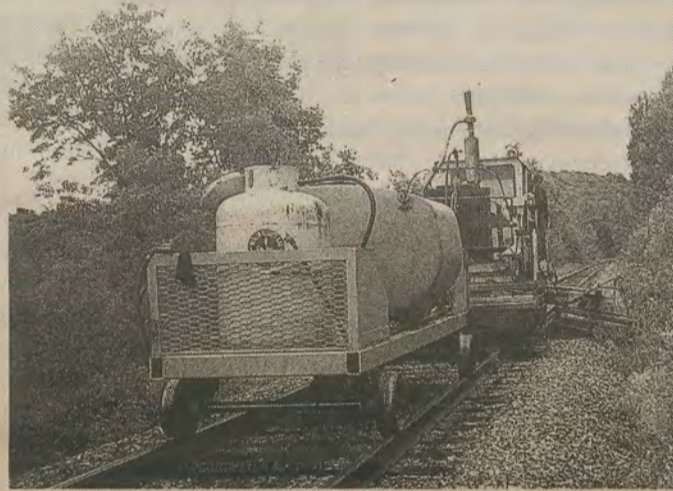
Track near Wenlock being treated in June with the retro-fitted equipment. Vegetation is watered, hit by hot air, and more water. Control extends 8' either side of the track. Photo © Barbara Alexander.
