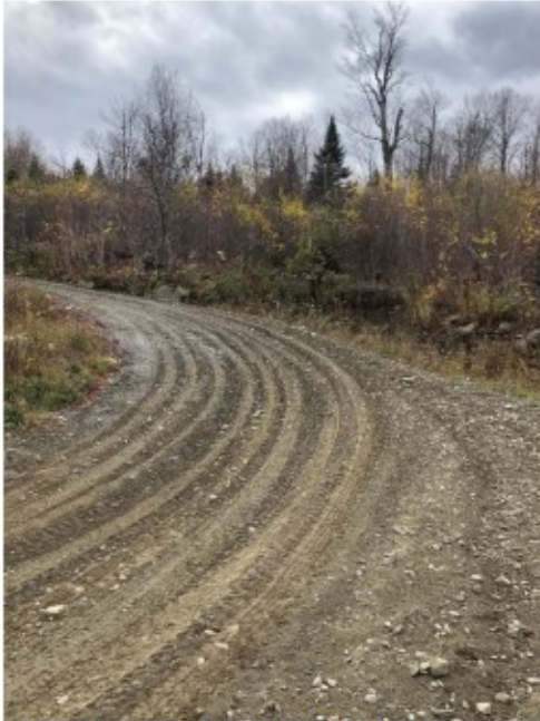
Figure 8- Shows berm on corner of trail
