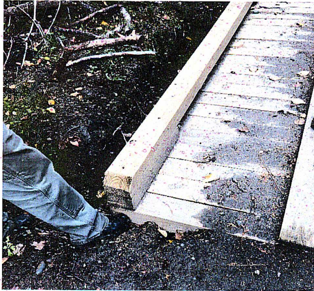
Figure 2- Minor sediment washing on edge of bridge
