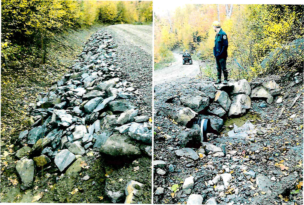
Figure 11 and 12- Depicts the newly fixed and armored ditch where the washout was previously. Also shows a newly installed culvert.
