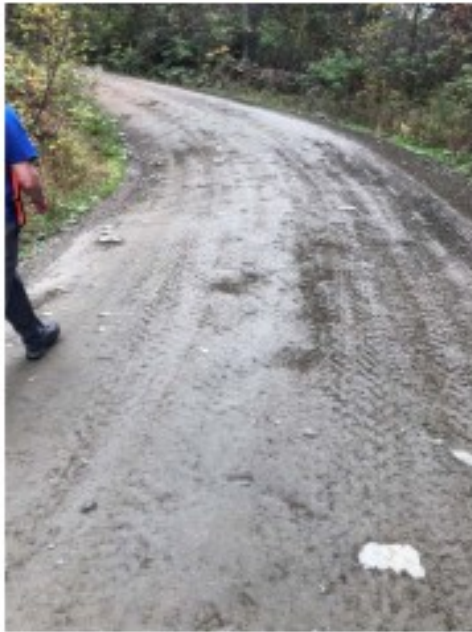
Figure 5- Shows condition of trail
