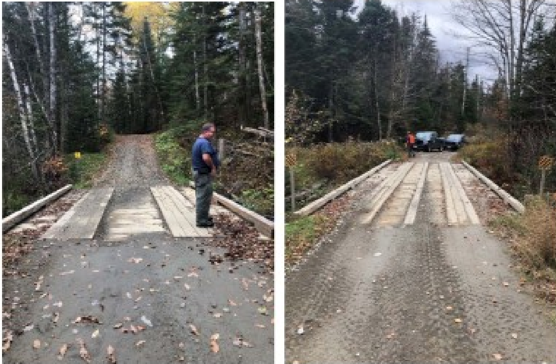
Figure 2- Shows the condition of the bridges
