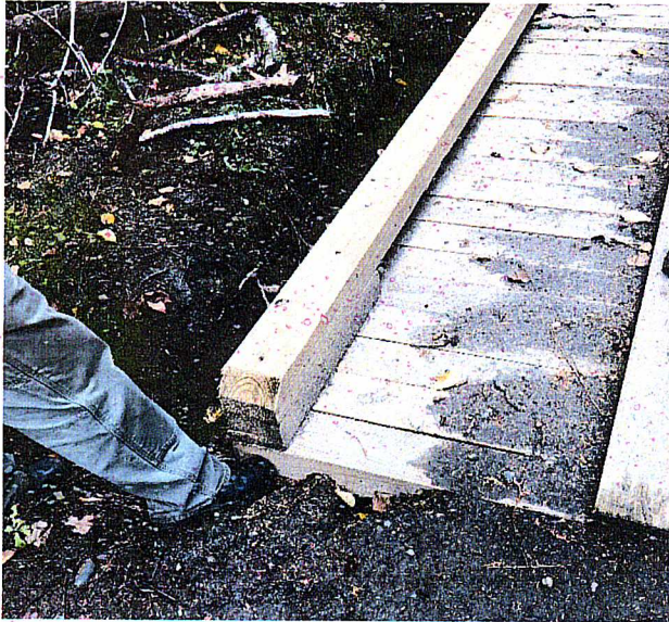
Figure 2- Minor sediment washing on edge of bridge
