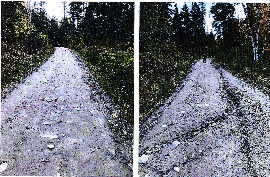
Figure 3- Shows condition of trail
