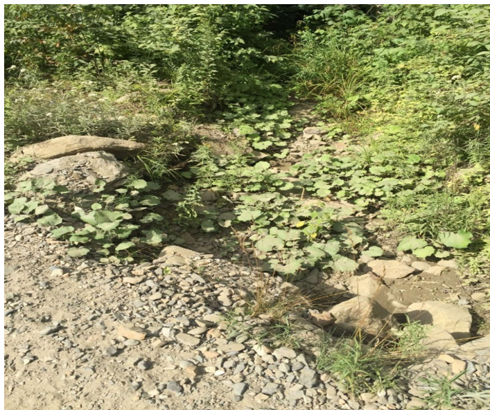
Drainage ditch with erosion and dust
