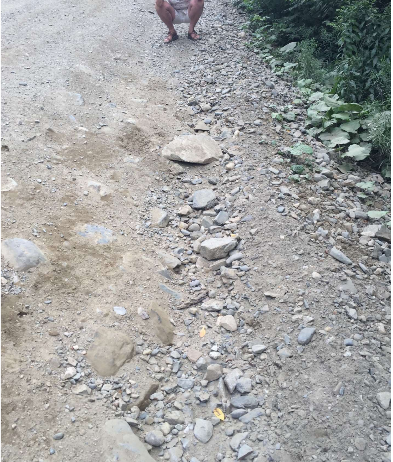
More erosion covered with new gravel spilling into ditch
