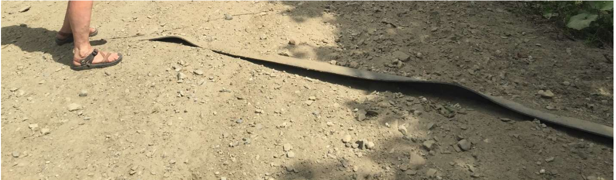
Ineffective Water Bar
