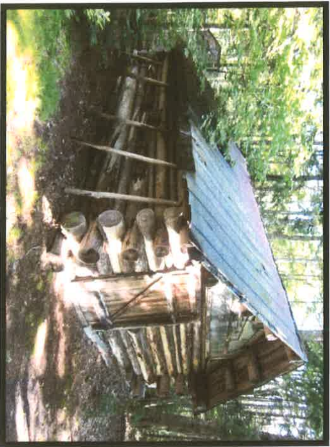
42. Large rotting cabin on Couture lease lot, facing NE
