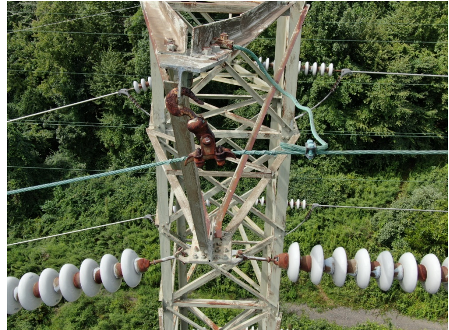
Lattice Tower Degradation – Structure #1348
