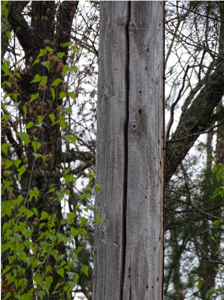
Typical Pole Split/Woodpecker Damage – Line C129
