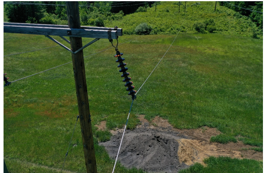
Typical Crossarm Damage – G128 Line
