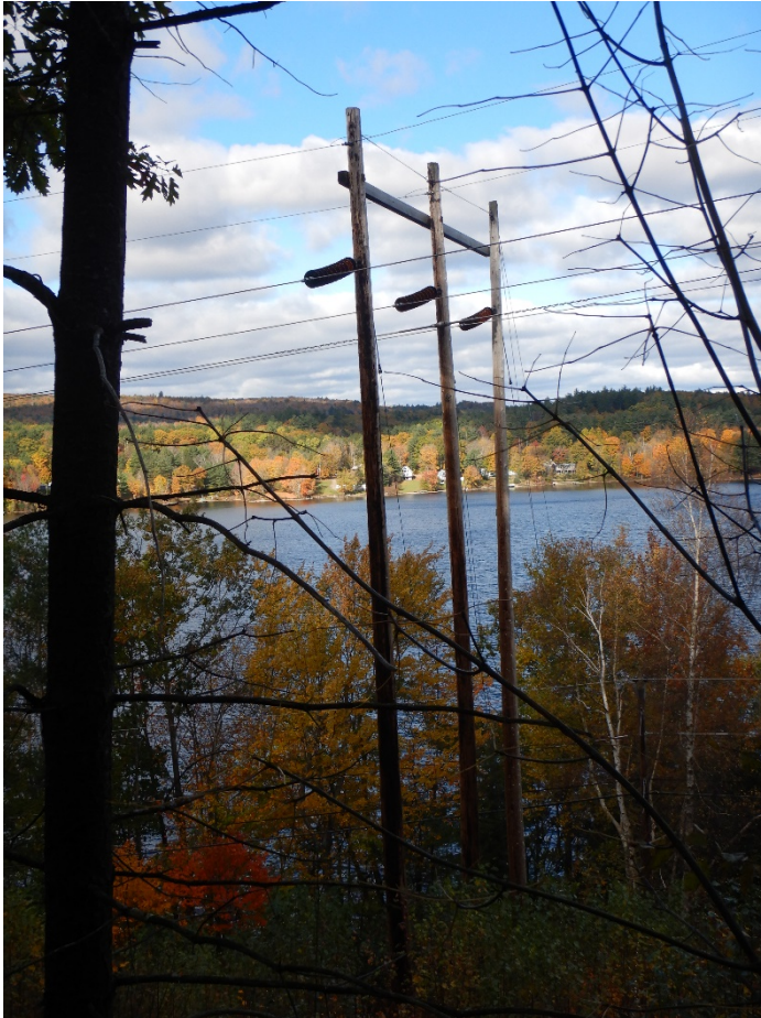
Typical Pole Splits/Woodpecker Damage – X104 Line
