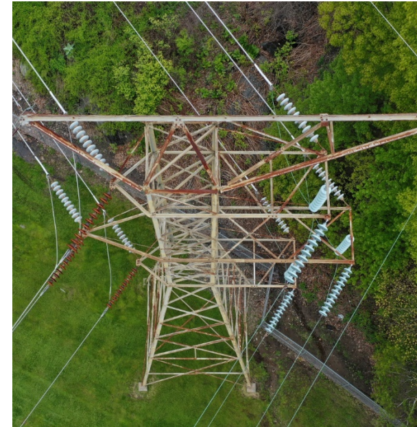
Rust on Steel, De-Galvanizing – Structure #8169
