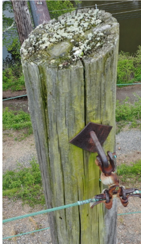
Split Pole Top, Woodpecker Damage – Structure #1847
