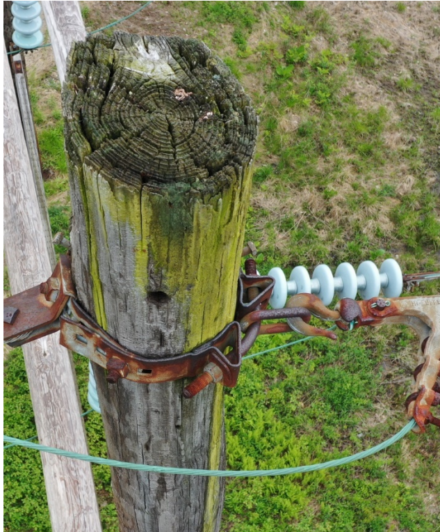
Rotten and Split Pole Top, Woodpecker Damage – Structure #1845
