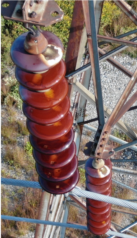
Damaged Flashed Insulators – Lattice Structure #25
