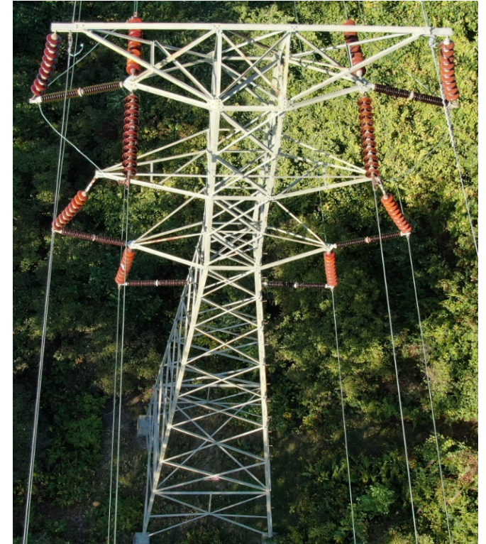
Existing Lattice Towers Built to 69-kV Spec
