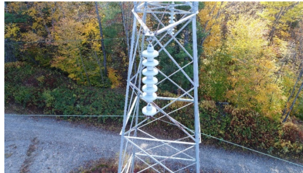
Structure 31231 – Missing Insulator Bell
