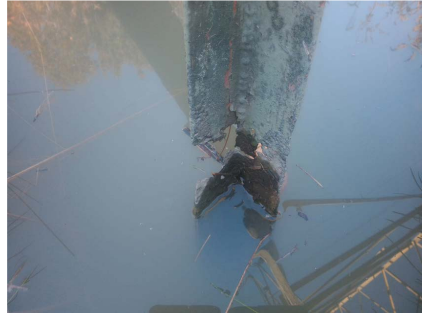
Lattice Tower Leg in Standing Water, Rusty and Eroding – Structure #248
