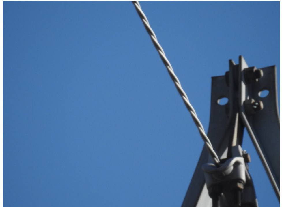
EHS Steel Shield Wire – Line C129
