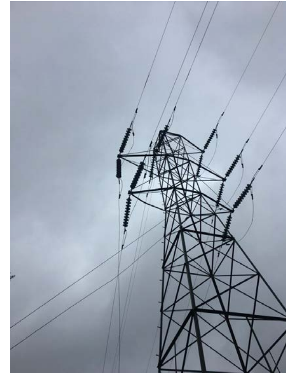
Broken Arm – Structure 31052
