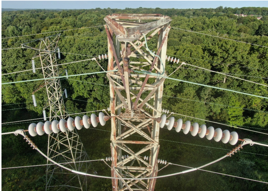
Lattice Tower Degradation – Structure #1362
