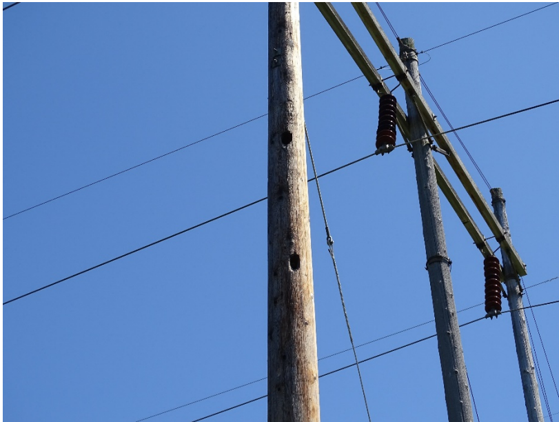
Typical Woodpecker Damage – G128 Line
