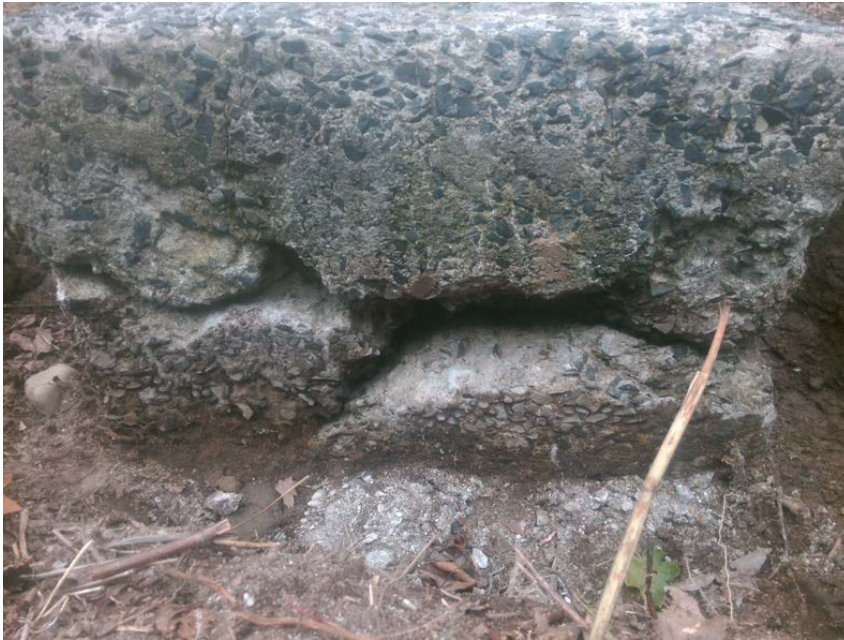
Damaged, Cracking, Crumbling Lattice Tower Leg Foundation – Structure #233
