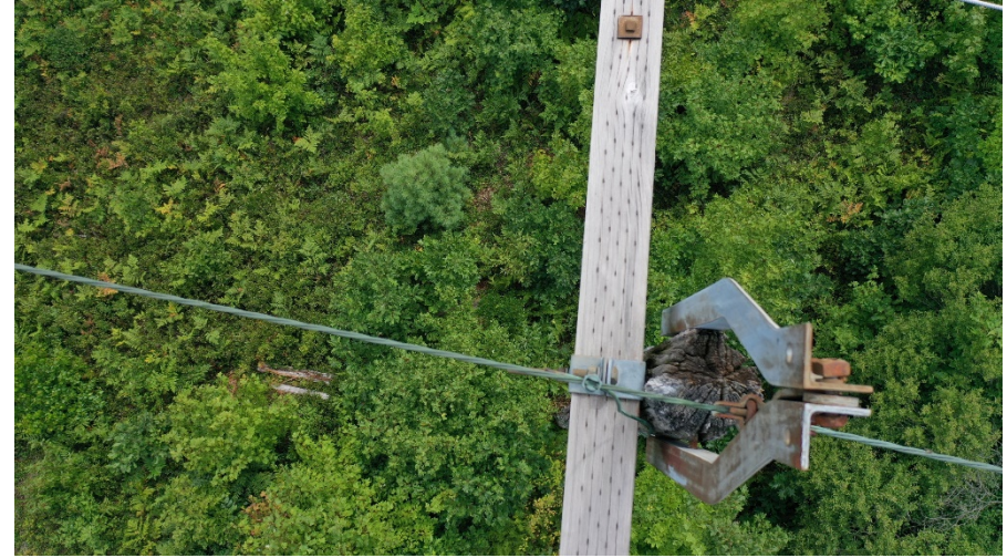
Pole Top Rot – Structure #65
