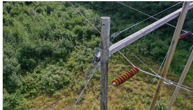
Pole Split – Structure #95
