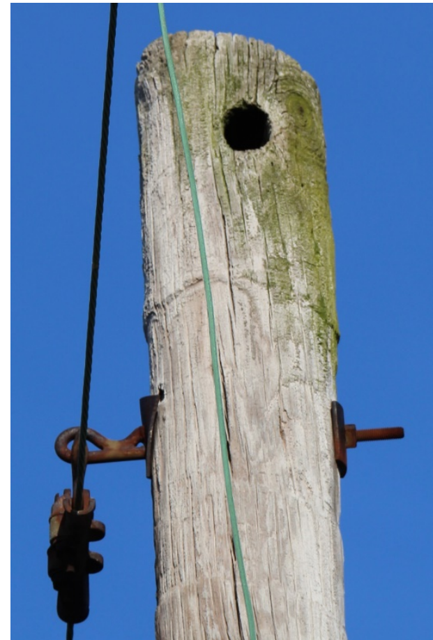
Split Pole Tops, Cracks and Woodpecker Damage – Structure #3624
