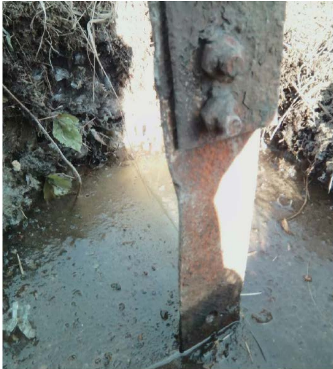
52.9% Section Loss of Leg Below Grade – Structure 31223
