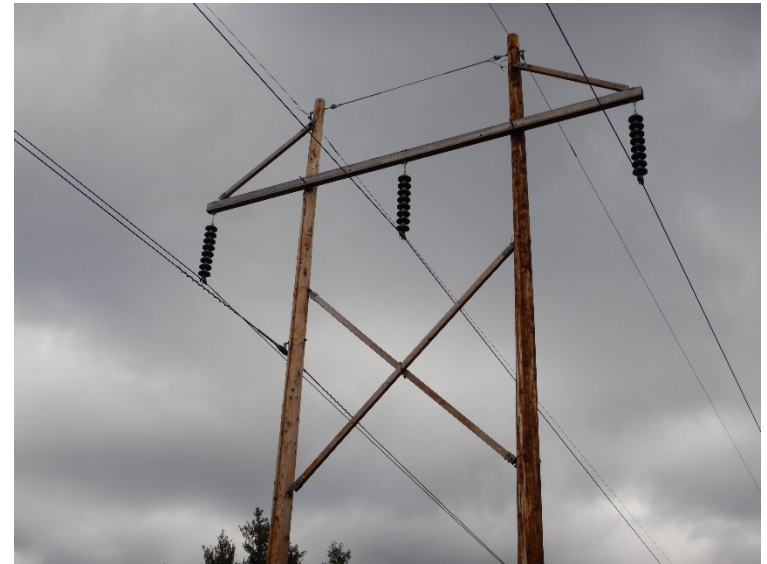
Typical Woodpecker Damage – X104 Line
