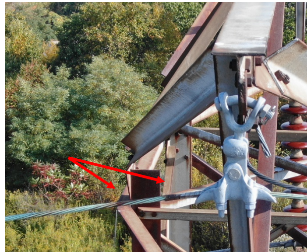
Corrosion of Copper Shield Wire
