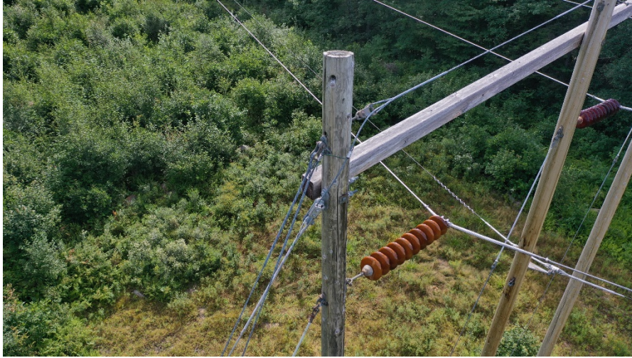
Pole Split and Woodpecker Damage – Structure #205
