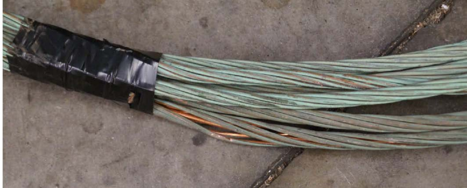
Damaged Strand of Existing 2/0 Copper Conductor Sample
