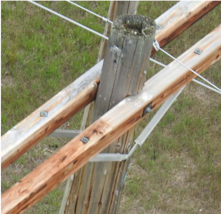
Pole Top Rot – Structure #284
