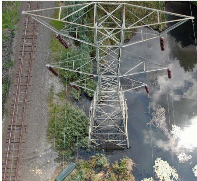
Lattice Structures in Standing Water and Wetlands Along Train Tracks Between Brookfield Jct and Structure #4620
