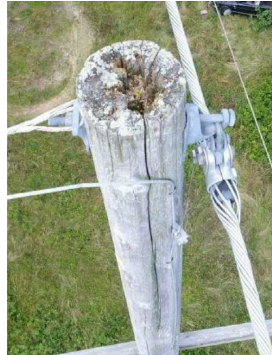
Line 191 Structure 27 – Age, Decay, Rotted Pole Tops
