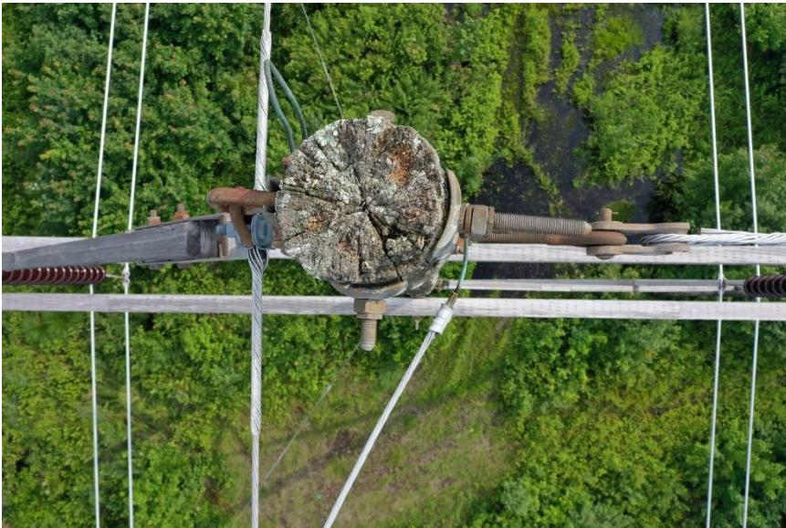
385 Line – Top Rot and Splitting
