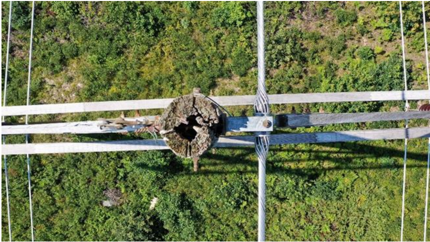
373 Line – Top Rot and Splitting
