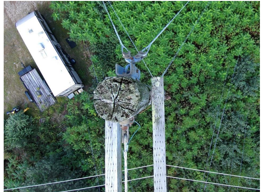
326 Line – Top Splitting and Cracking
