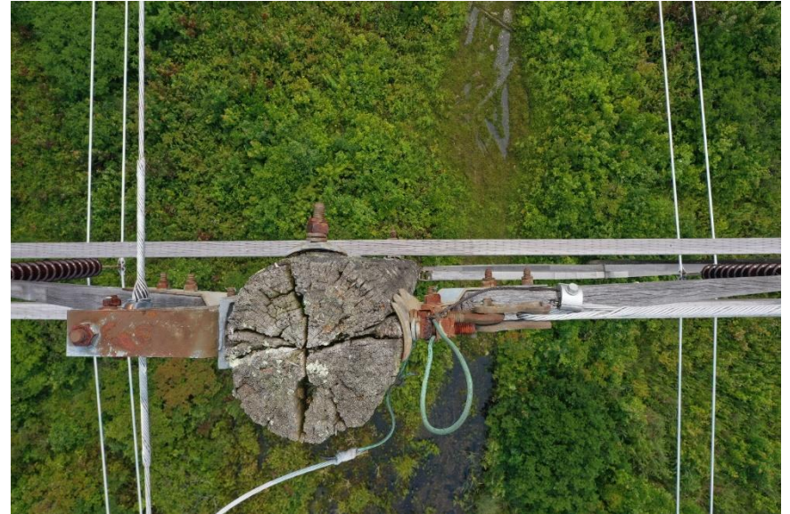
391 Line – Top Splitting and Cracking
