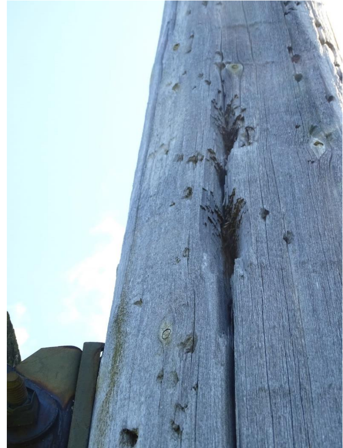
379 Line – Pole Splitting and Woodpecker Damage
