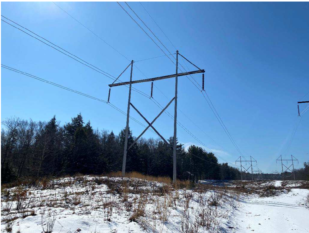
Photograph No. 42: Looking at proposed access and work pad location for 391 Structure 116.
