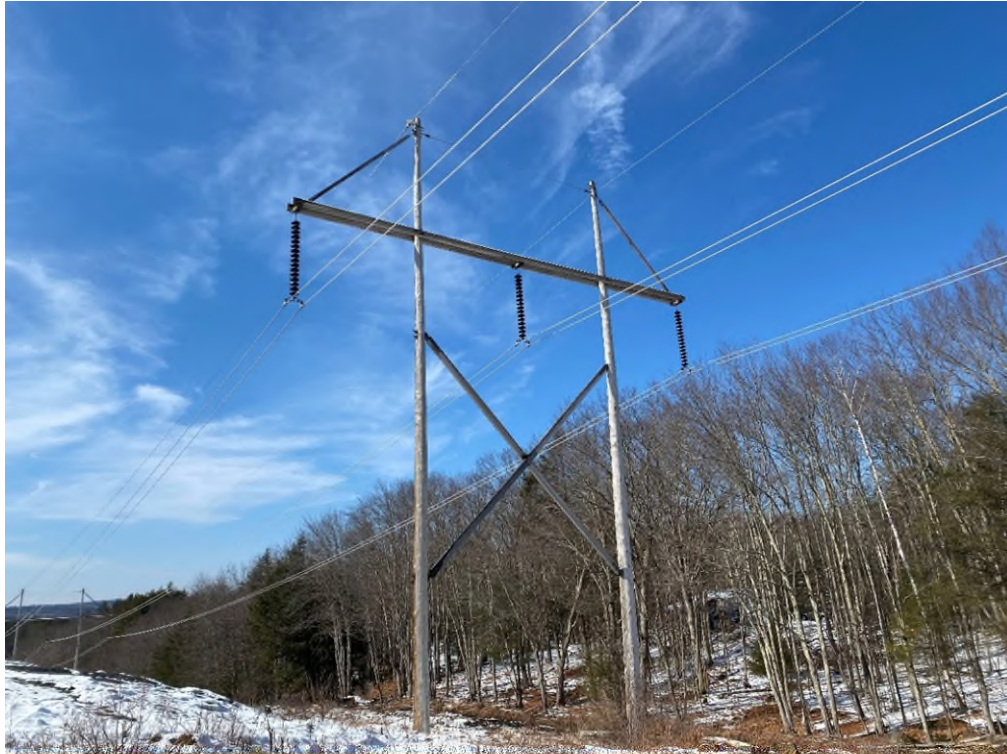
Photograph No. 47: Looking at proposed access and work pad location for 391 Structure 71.
