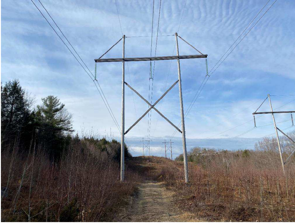
Photograph No. 25: Looking at proposed access and work pad location adjacent to 391 Structure 192.
