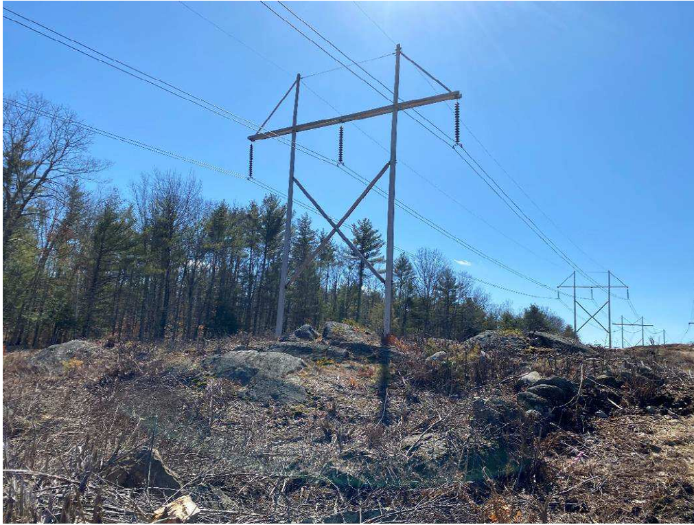
Photograph No. 55: Looking at proposed access and work pad location for 391 Structure 72.
