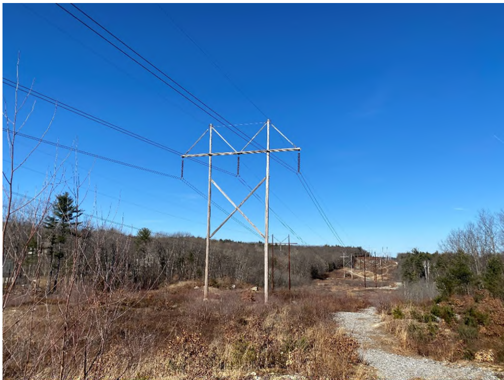
Photograph No. 16: Looking at proposed access and work pad location adjacent to 391 Structure 272.
