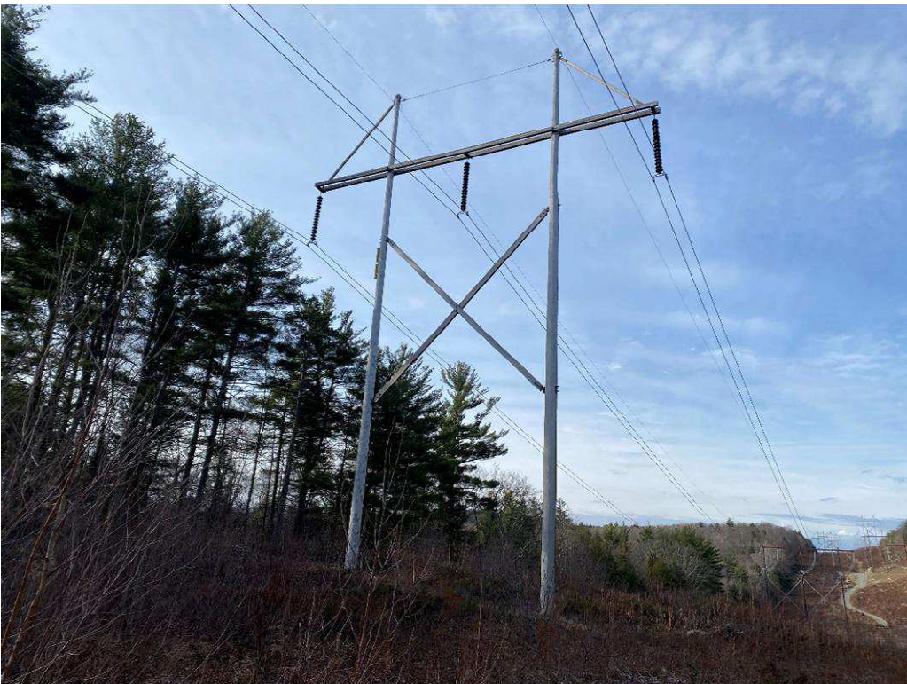
Photograph No. 28: Looking at proposed access and work pad location for 391 Structure 177 from Nottingham Road.
