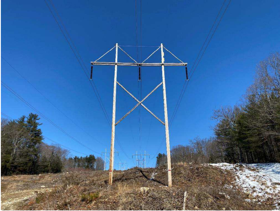
Photograph No. 37: Looking at proposed access and work pad location for 391 Structure 131.
