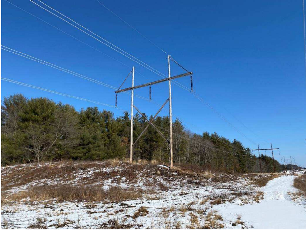
Photograph No. 43: Looking at proposed access and work pad location adjacent to 385 Structure 80.
