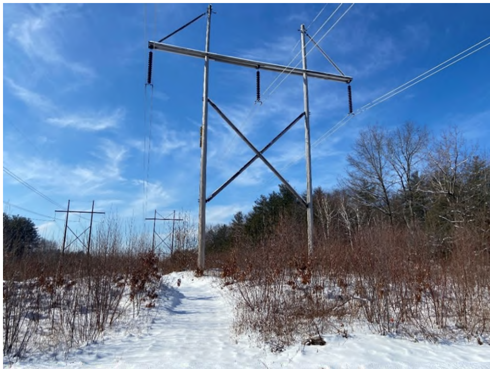
Photograph No. 2: Looking at proposed access and work pad location for 373 Structure 320.
