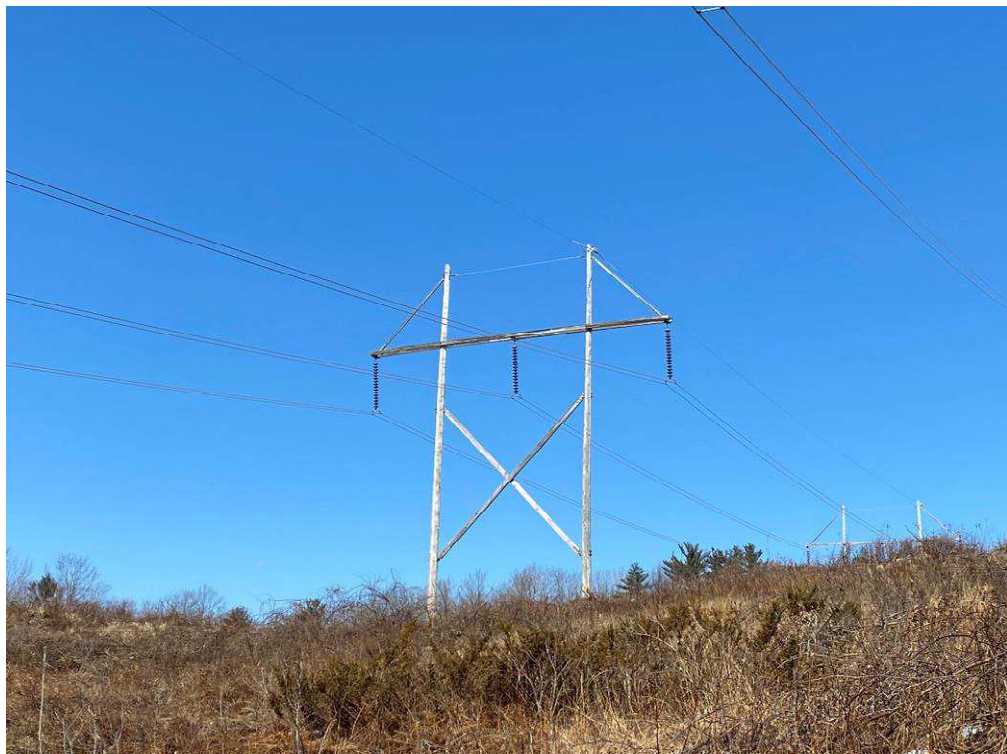
Photograph No. 40: Looking at proposed access and work pad location for 385 Structure 125.
