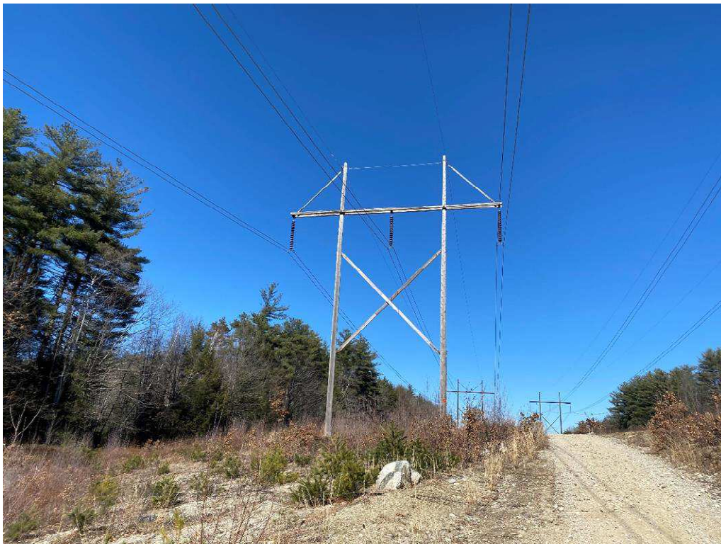
Photograph No. 24: Looking at proposed access and work pad location for 373 Structure 235.
