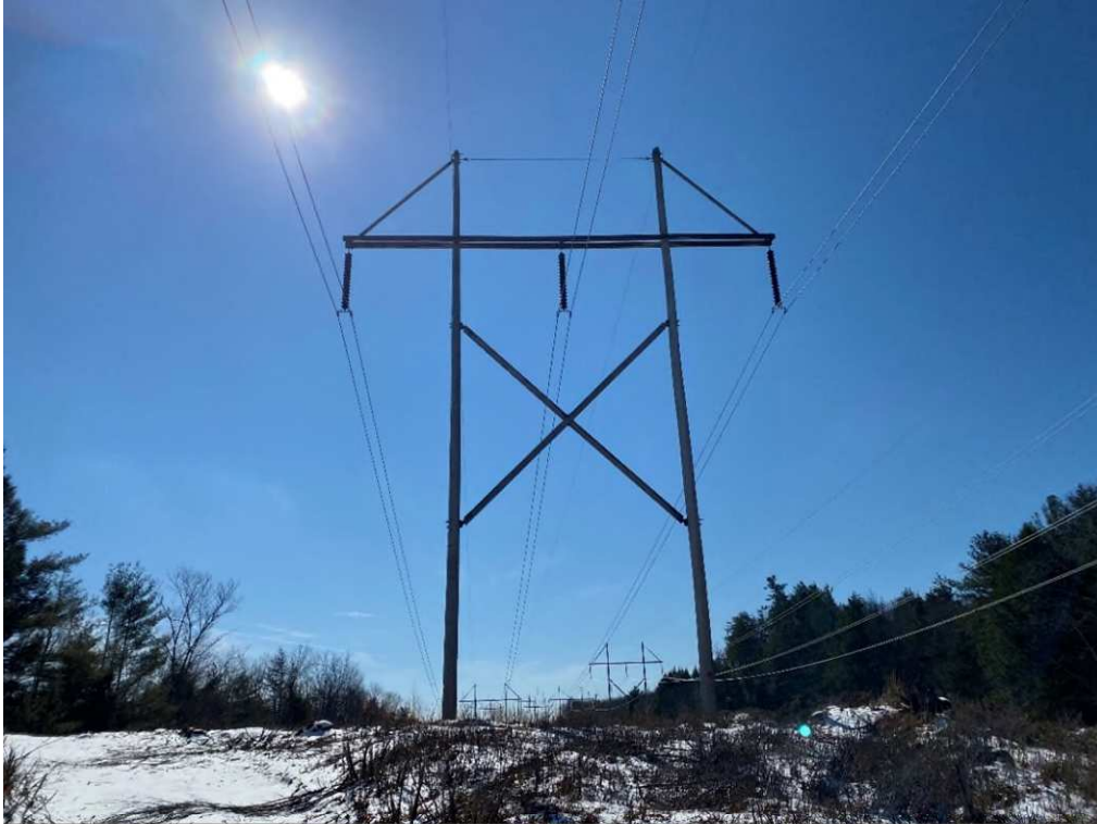
Photograph No. 35: Looking at proposed access and work pad location for 391 Structure 132.
