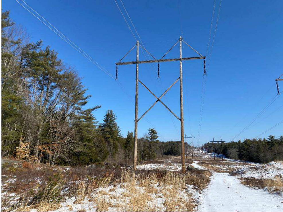
Photograph No. 45: Looking at proposed access and work pad location for 385 Structure 77.
