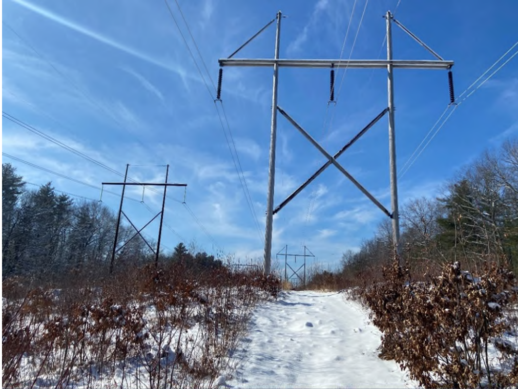
Photograph No. 5: Looking at proposed access and work pad location for 373 Structure 317.
