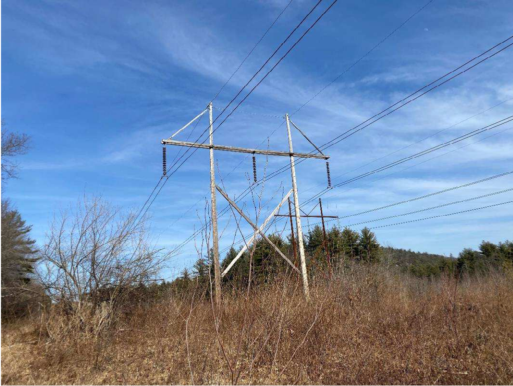
Photograph No. 23: Looking at proposed access and work pad location for 373 Structure 246.
