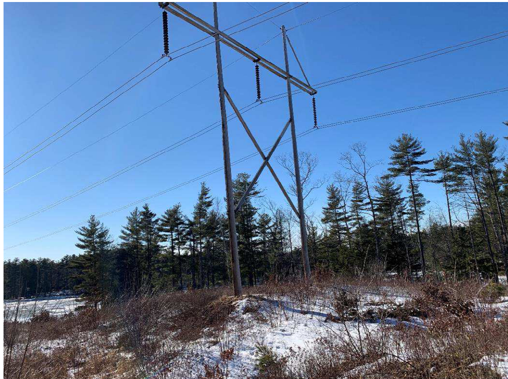
Photograph No. 14: Looking at proposed access and work pad location adjacent to 391 Structure 274.
