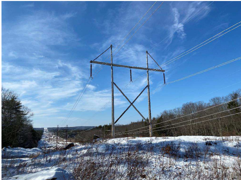
Photograph No. 48: Looking at proposed access and work pad location for 391 Structure 78.
