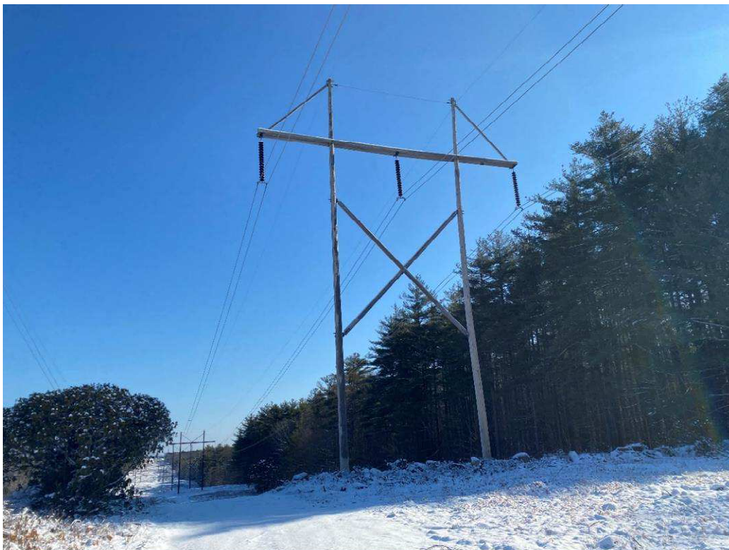
Photograph No. 60: Looking at proposed access and work pad location for 391 Structure 46.
