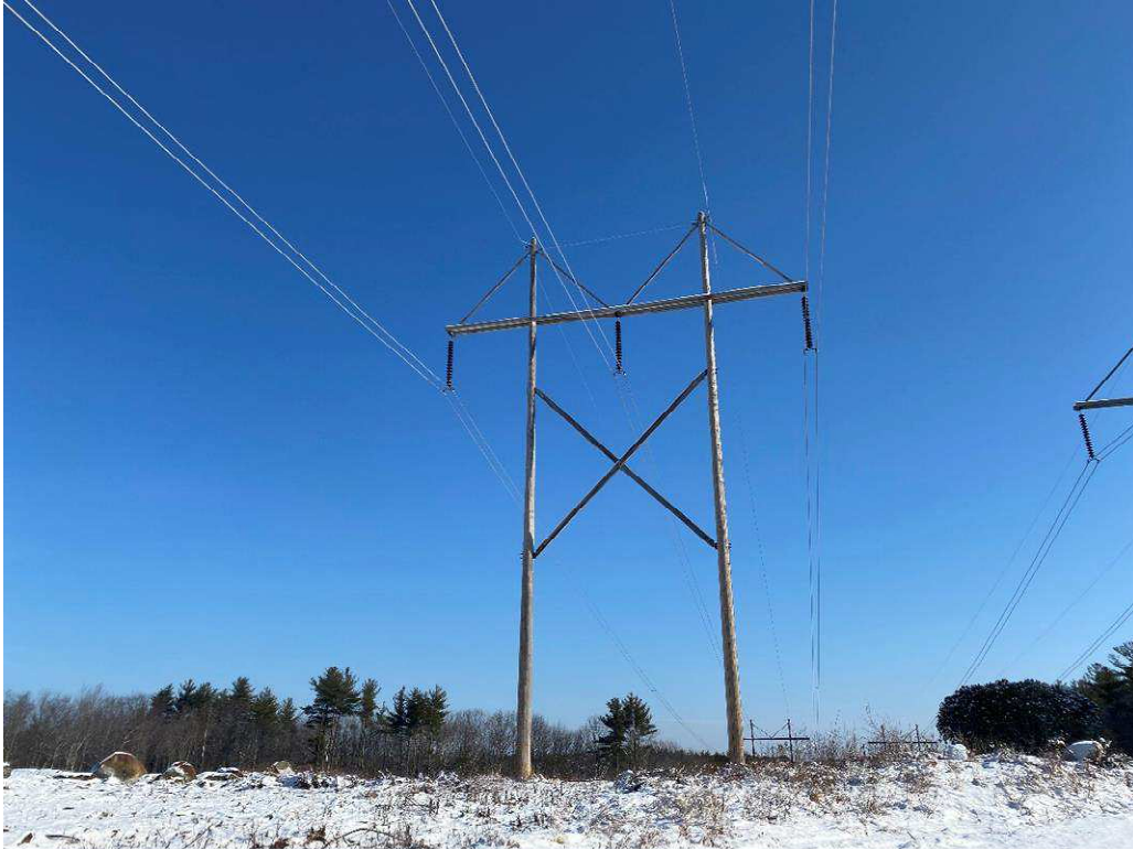
Photograph No. 59: Looking at proposed access and work pad location for 385 Structure 43
