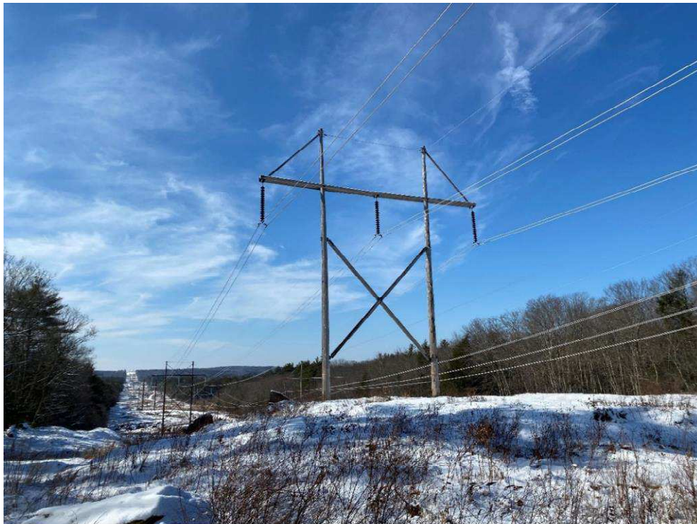
Photograph No. 46: Looking at proposed access and work pad location for 385 Structure 72.
