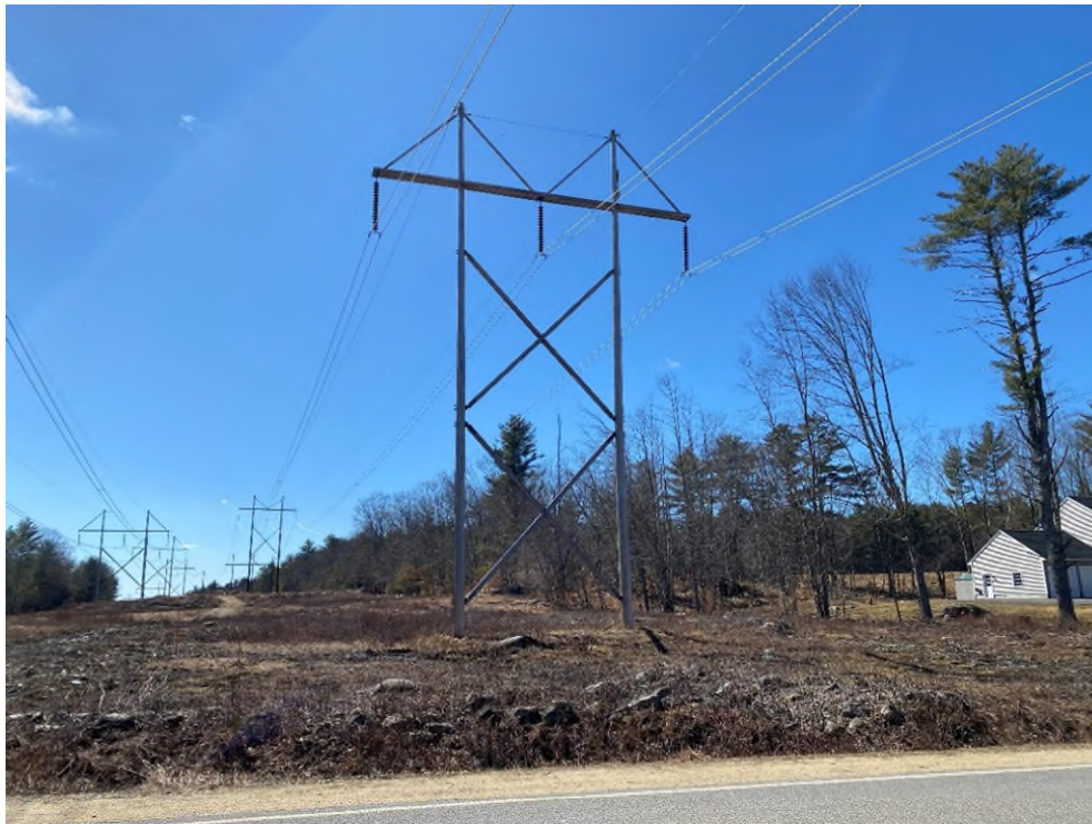
Photograph No. 56: Looking at proposed access and work pad location to 385 Structure 65 from Second Crown Point Road.
