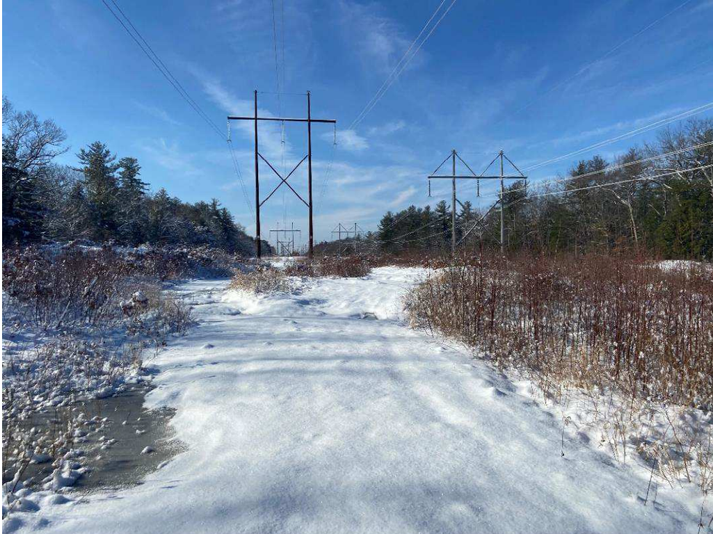
Photograph No. 7: Looking at proposed access and work pad location from Pingree Hill Road for 373 Structure 126.
