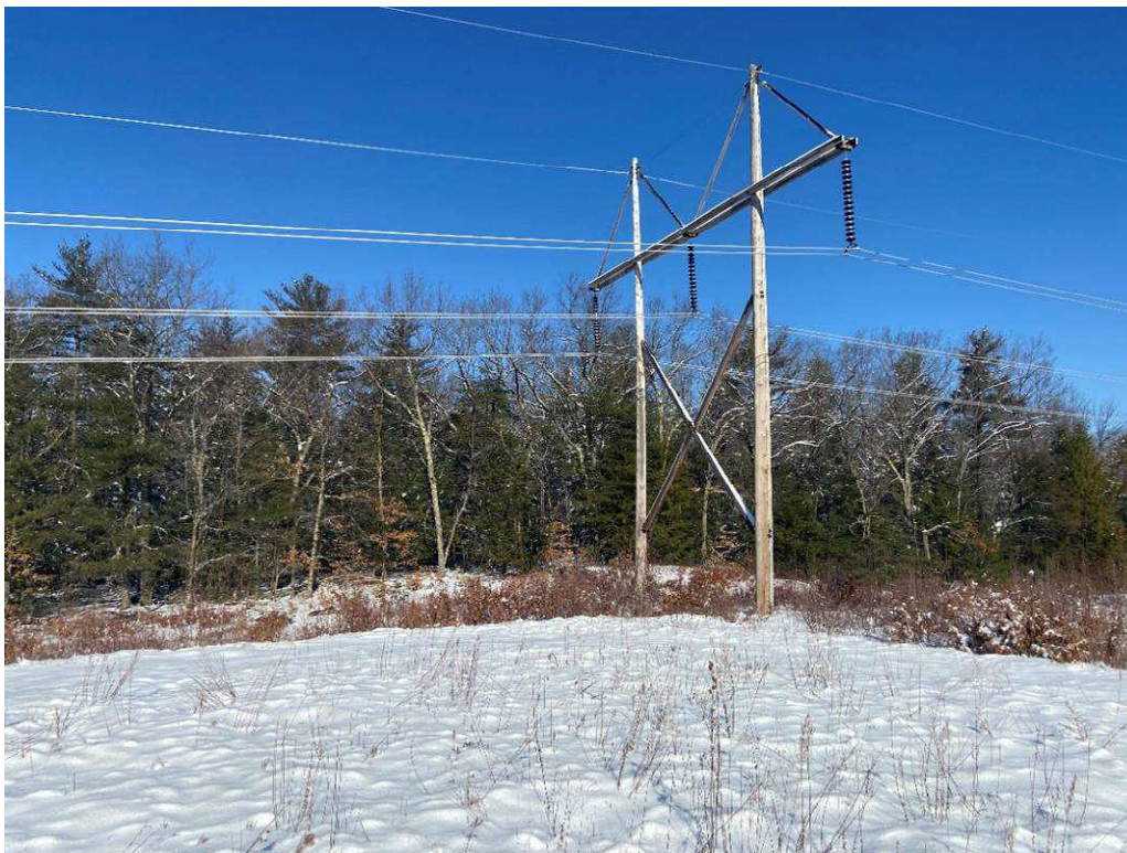
Photograph No. 6: Looking at proposed access and work pad location adjacent to 373 Structure 316.
