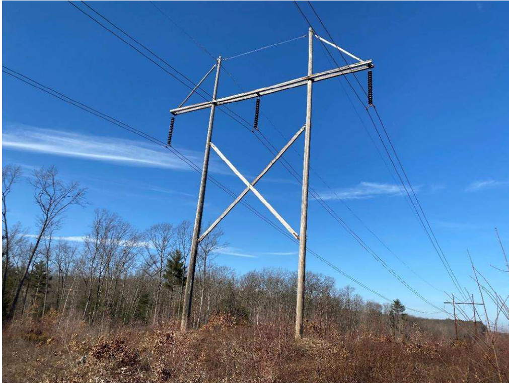
Photograph No. 15: Looking at proposed access and work pad location adjacent to 373 Structure 275.
