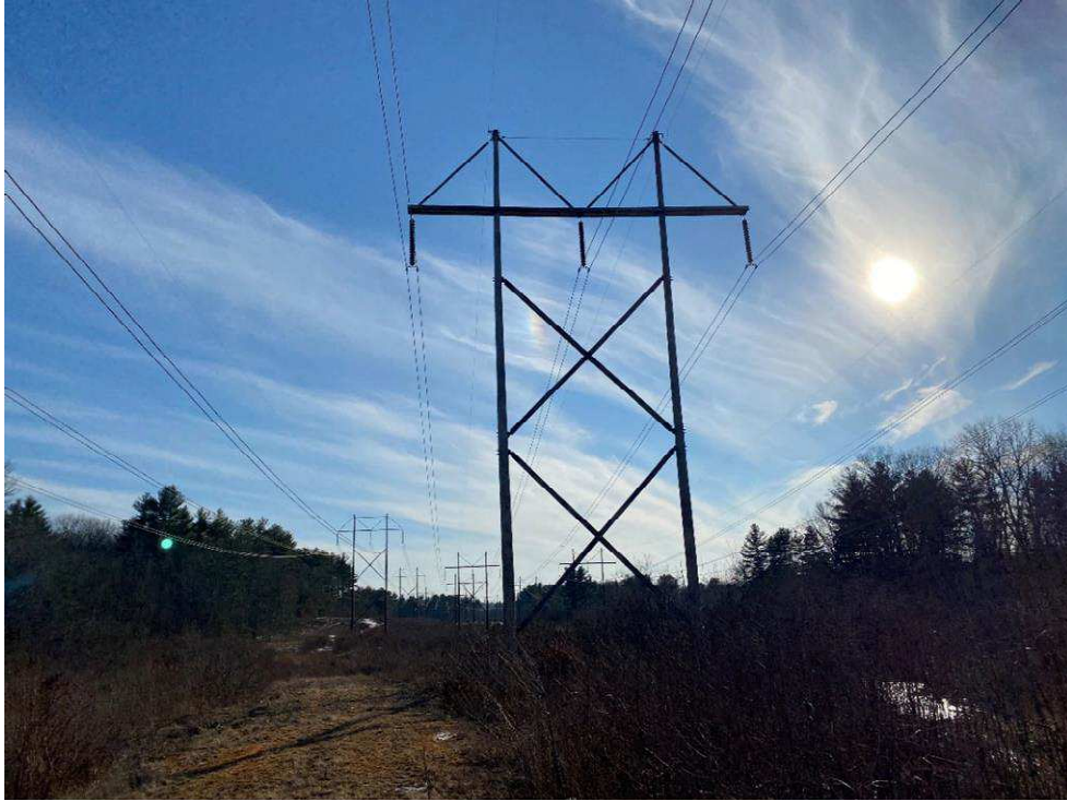
Photograph No. 1: Looking at proposed access and work pad location from Route 28 to 391 Structure 326.
