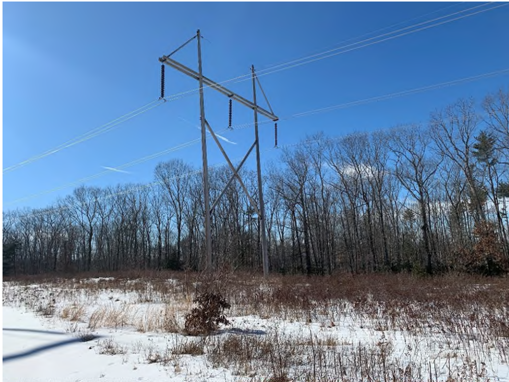
Photograph No. 12: Looking at proposed access and work pad location adjacent to 373 Structure 295.
