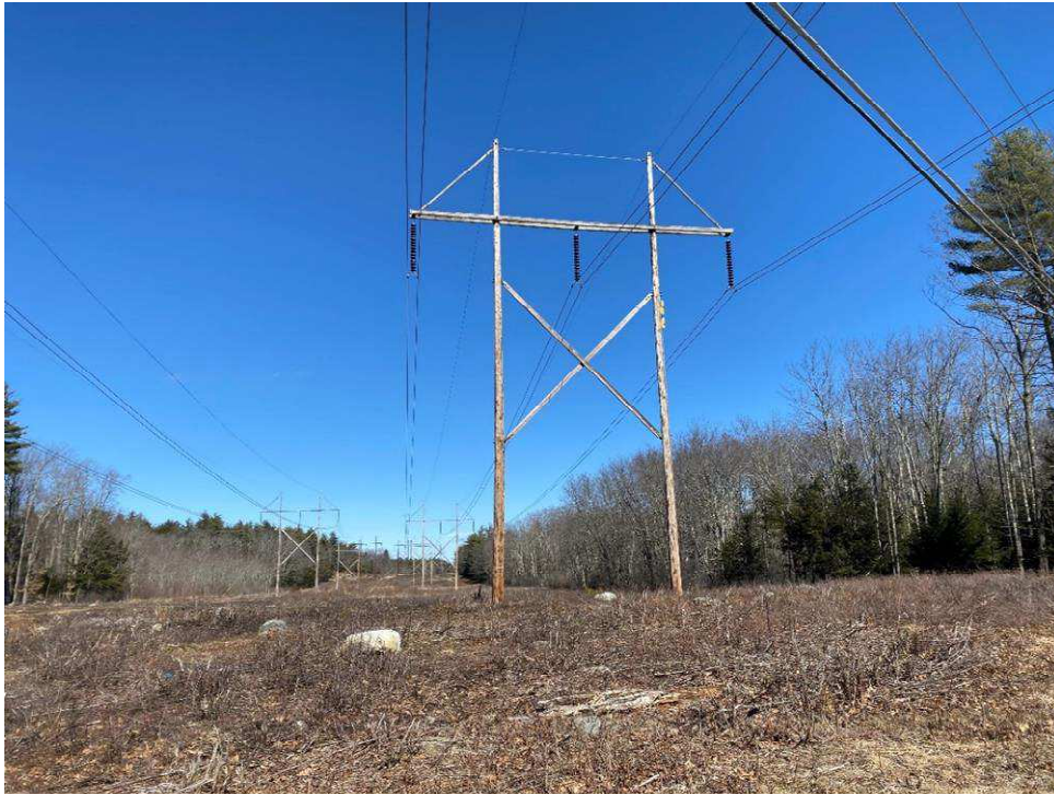
Photograph No. 49: Looking at proposed access and work pad location for 391 Structure 77.
