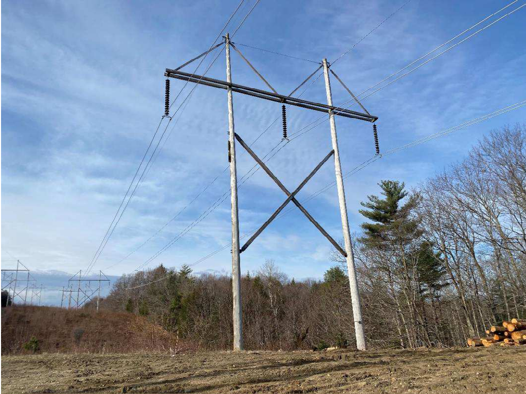
Photograph No. 27: Looking at proposed access and work pad location adjacent to 373 Structure 186.
