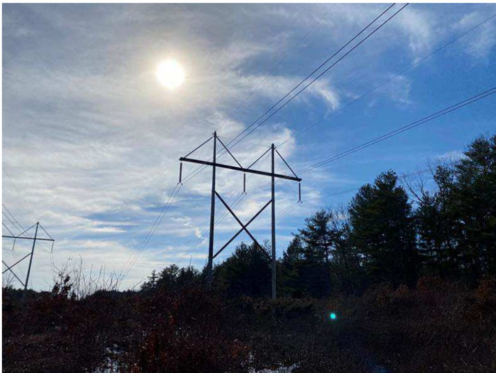
Photograph No. 18: Looking at proposed access and work pad location adjacent to 373 Structure 263.
