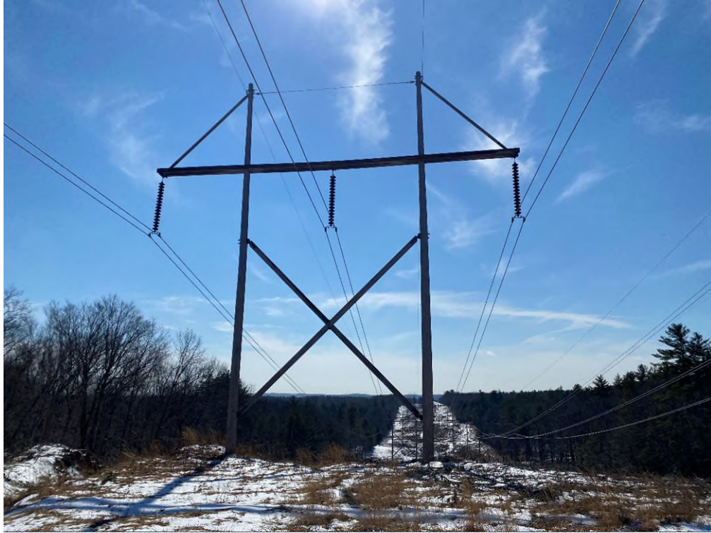
Photograph No. 39: Looking at proposed access and work pad location for 391 Structure 130.
