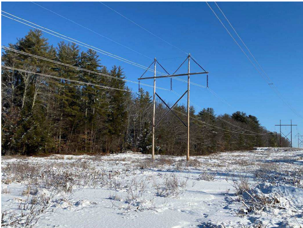
Photograph No. 62: Looking at proposed access and work pad location for 385 Structure 33.
