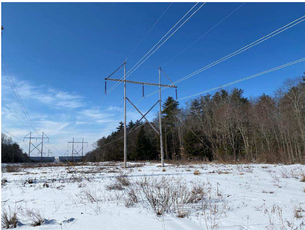
Photograph No. 50: Looking at proposed access and work pad location adjacent for 385 Structure 69.
