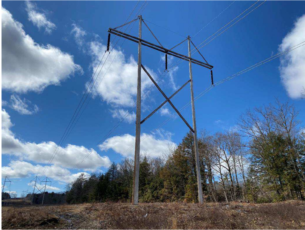
Photograph No. 63: Looking at proposed access and work pad location for 385 Structure 23.
