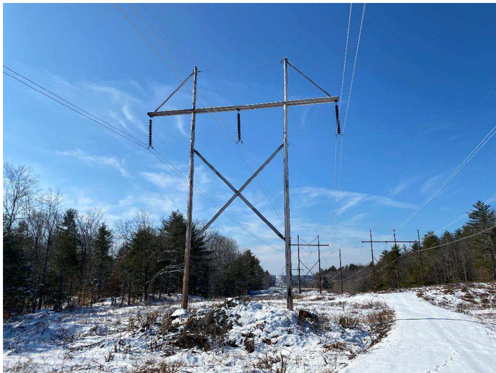
Photograph No. 54: Looking at proposed access and work pad location for 391 Structure 73.
