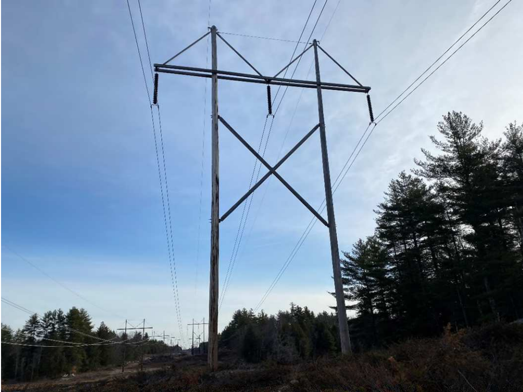
Photograph No. 29: Looking at proposed access and work pad location for 391 Structure 163.
