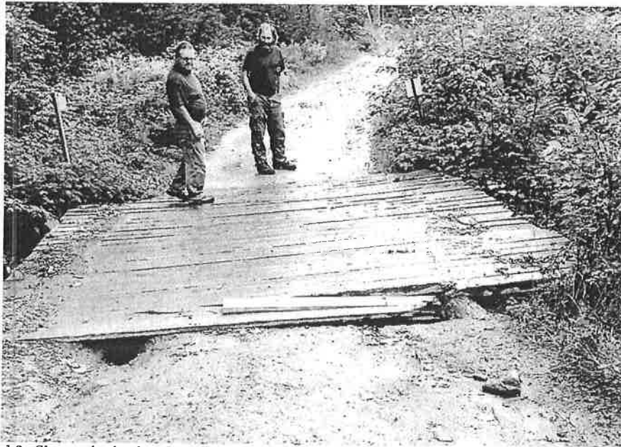
Figure 1, 2 and 3- Shows the broken boards on the bridges and the eroding approaches.
