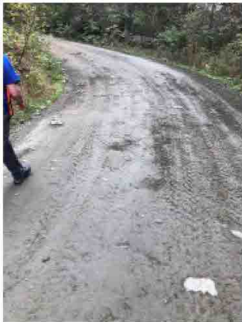
Figure 5- Shows condition of trail
