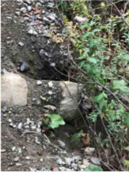
Figure 6- Depicting the area where the water is eroding around the culvert.
