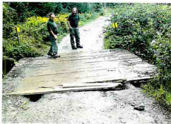
Figure 1, 2 and 3- Shows the broken boards on the bridges and the eroding approaches.
