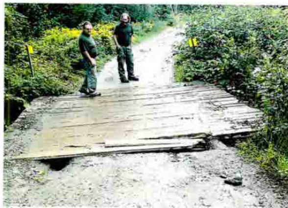
Figure 1, 2 and 3- Shows the broken boards on the bridges and the eroding approaches.
